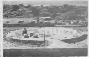
SAND IS needed to form a solid packed base. Depending on the elevation of the site up to 10 feet of sand was poured.
